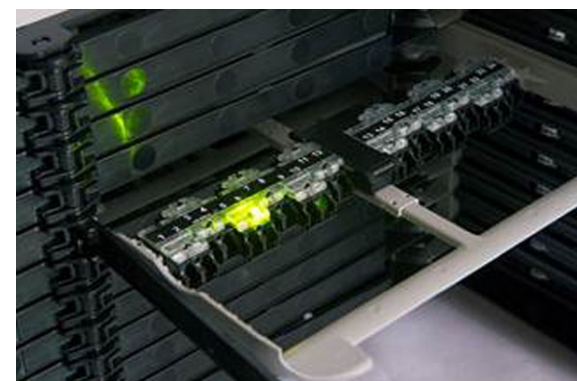
CPID chips embedded in a patch panel.
